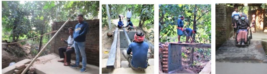
Workers' masters: Binay, Novin...our carpenter Anondo ... I test the strength!!! All the beams and planks are made with the wood of our crushed trees. Masonry is still not completed.
